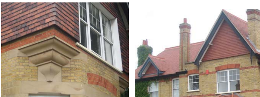
Retention of some stone detailing, but loss of joinery detail to the gables at restoration
