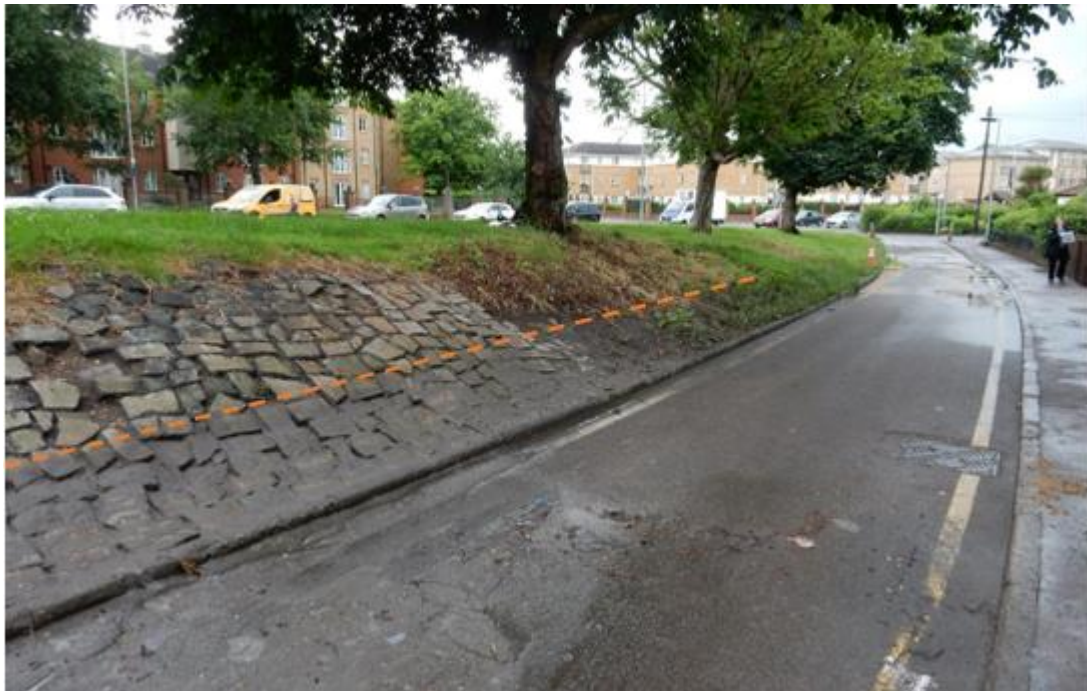
Figure 24: Photo taken at 4:43pm on Steven Jewers Gardens. Looking northwest towards the junction with Westrow Drive. Strong odour on site. Evidence of flooding from silt remnants in road. Note water line on stone banking, (orange line) approximately 0.5-0.7m up from road level.
